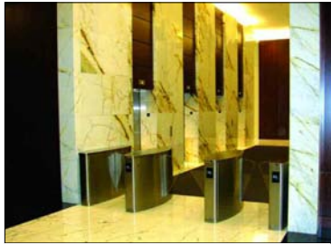
Electronic turnstiles, 225 Franklin Street
