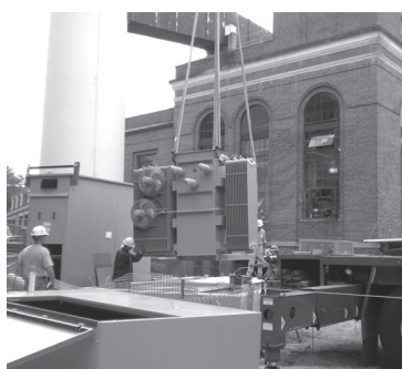
Padmount transformer which steps up supplemental generator voltage from 5kV to 38kV and interconnects to the Public Service power line, being offloaded for installation at UNH heating plant facility.
