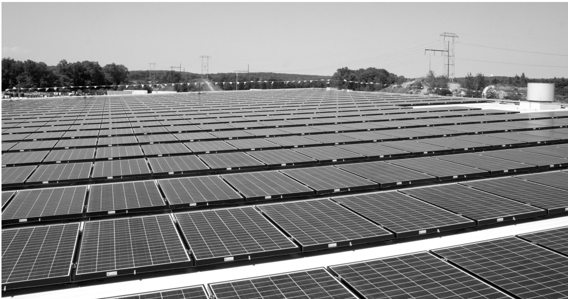
The 1MW solar generation facility at the National Grid New England Distribution Center warehouse in Whitinsville is the state's largest solar site.
