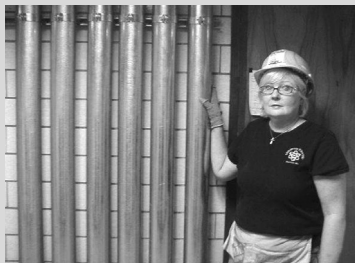
Maureen Thompson, principal of Maureen Electrical, shown after raceway installations at a UMass Boston project.
