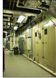
Special Air Handling Units
