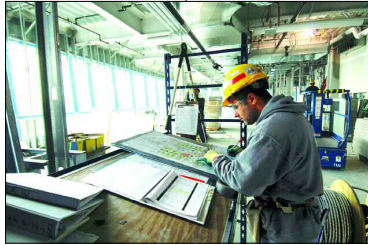
MEC electrician reviewing electrical drawing detail
