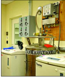
Installations for 140 Nitrogen Freezers
